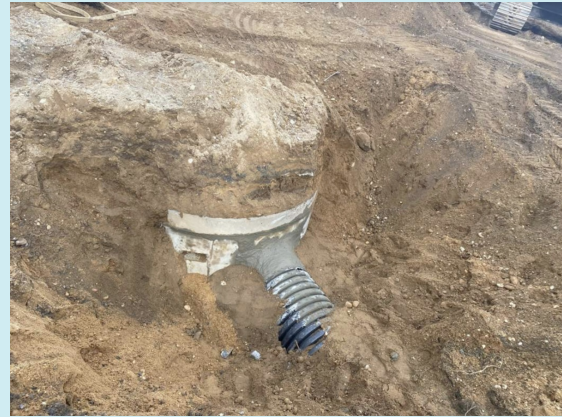
Permanent leeching pool for drainage
